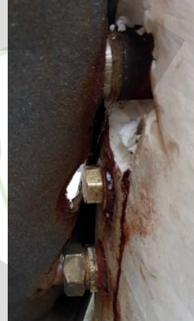
Electrochemical corrosion of steel tank connections „connected” with copper pipes can cause leakage after 16 months of operation, in the welding seams of the connections already within the first year of operation.
