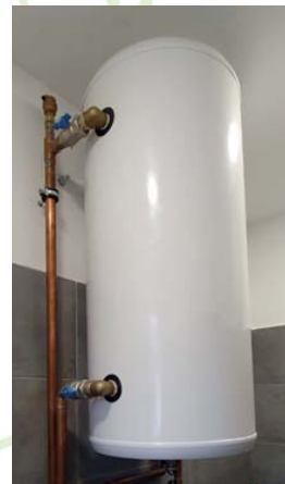
Hot water tank connected with a copper pipe, missing: tank grounding and dielectric common screw (plus expansion tank).
