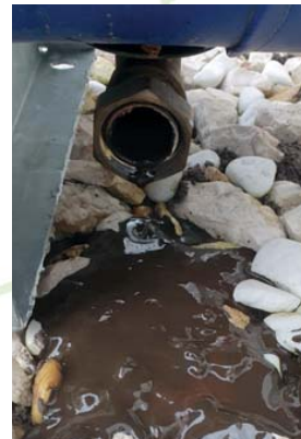
Rust sludge, this is the result of electrochemical and oxidative corrosion.
