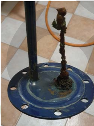
One of the consequences of electrochemical corrosion is rapid anode loss, which is why the first anode replacement is justified at 12 months, so in case of significant loss, the problem can be identified in time without damaging the storage body (18 months after that).
