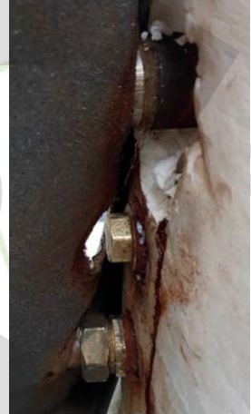
Electrochemical corrosion of steel tank connections „connected” with copper pipes can cause leakage after 16 months of operation, in the welding seams of the connections already within the first year of operation.
