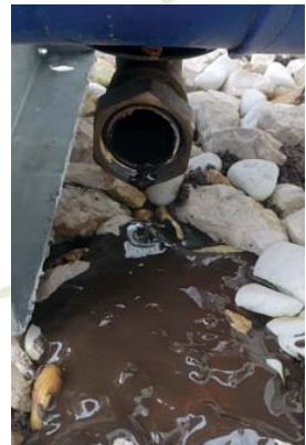
Rust sludge, this is the result of electrochemical and oxidative corrosion.
